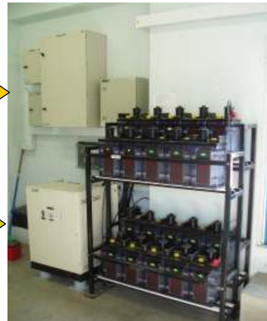
Energy storage and management
