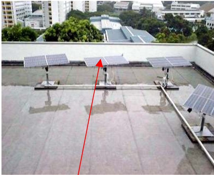
Singapore first Solar system installed in Singapore Polytechnic in 1993
