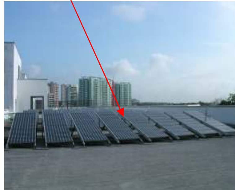
Singapore first large solar system installed in Singapore Polytechnic in 1996
